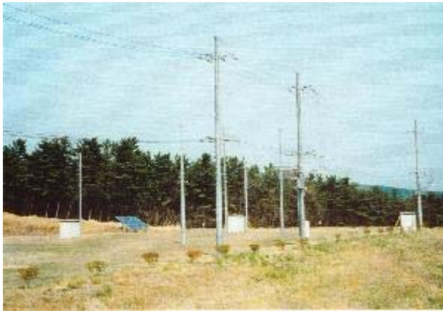
Facility for evaluation of radiated emission (Example of utilities interconnection)
